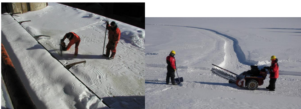
Figure 5. Cutting slots in the ice upstream of a spillway to minimize static ice loads on spillway gates. (Photo: Manitoba Hydro)
