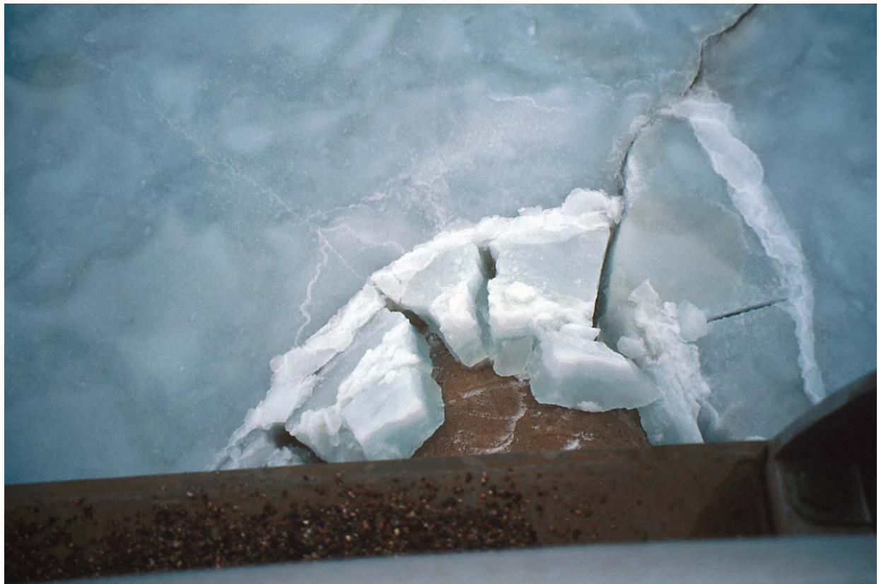
Fig. 7. Ride-up of ice wedges formed by radial and circumferential cracks on a pier of the Upper Blackville bridge. Fracture pattern is typical of bending failure.
