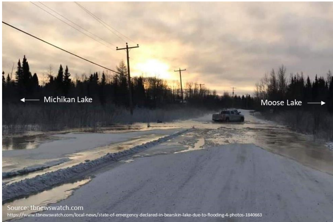
Figure 5. Photograph of overtopped road at Moose River Crossing
