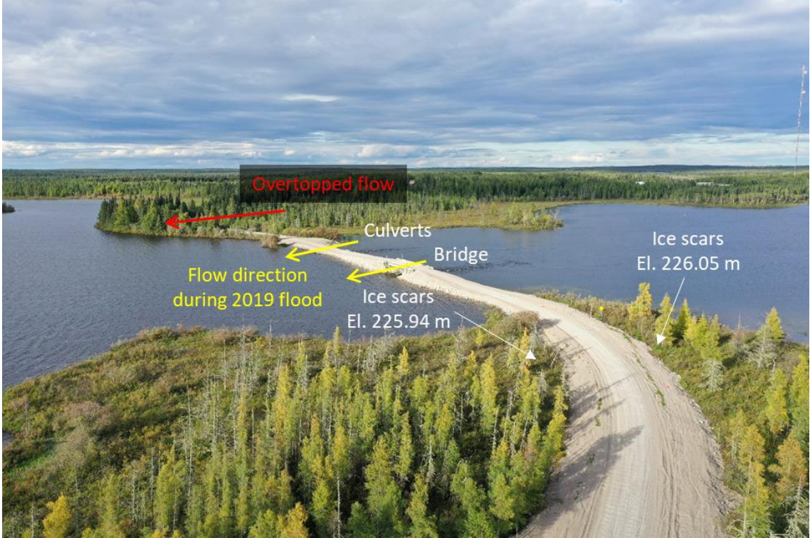
Figure 8. Flood impacts at Mahan Bridge – Photo A
