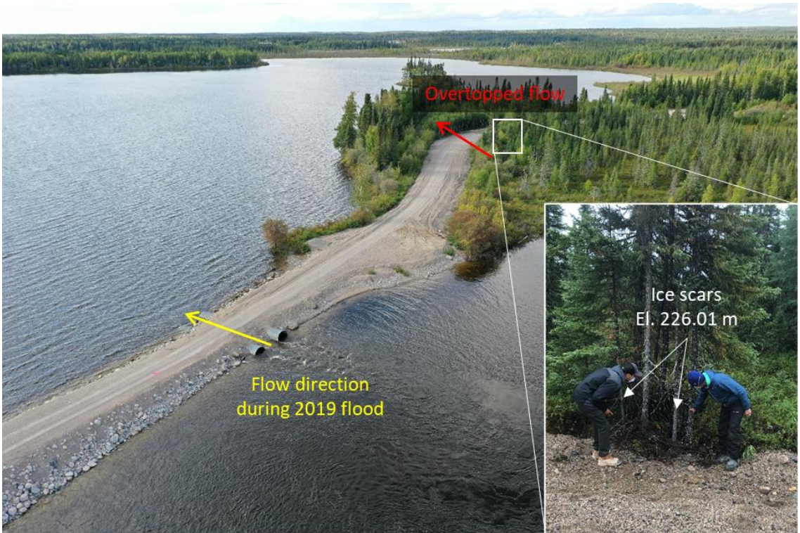
Figure 9. Flood impacts at Mahan Bridge – Photo B
