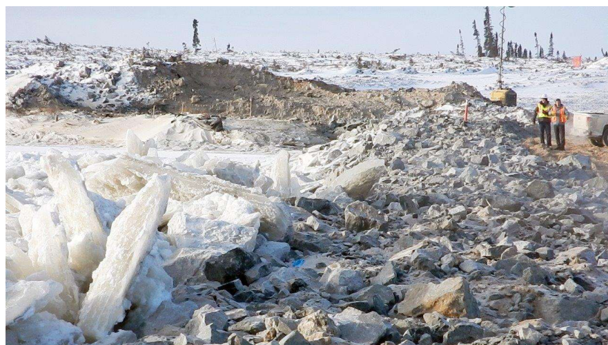
Figure 8: Accumulating Ice at Crest of the Powerhouse Cofferdam
