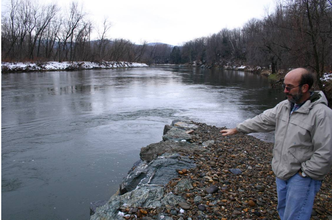
Fig. 3. Ice resistant rock vane designed and built by the Vermont NRCS to stabilize an eroding bank along the Winooski River near Richmond, VT.
