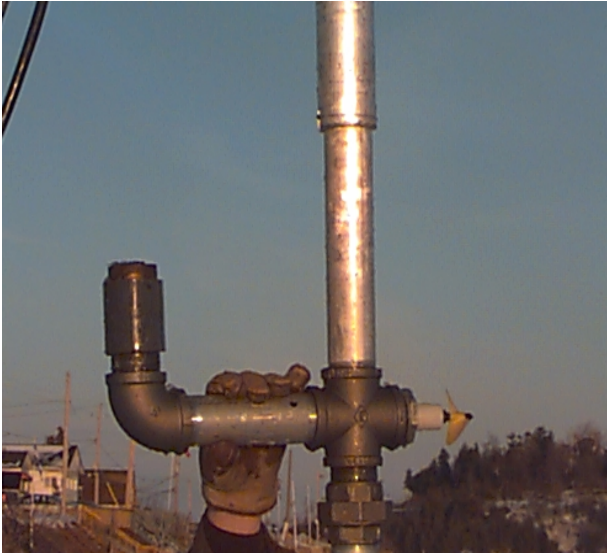
Figure 1. Instrument Assembly Used for the Mackenzie Measurement Project
